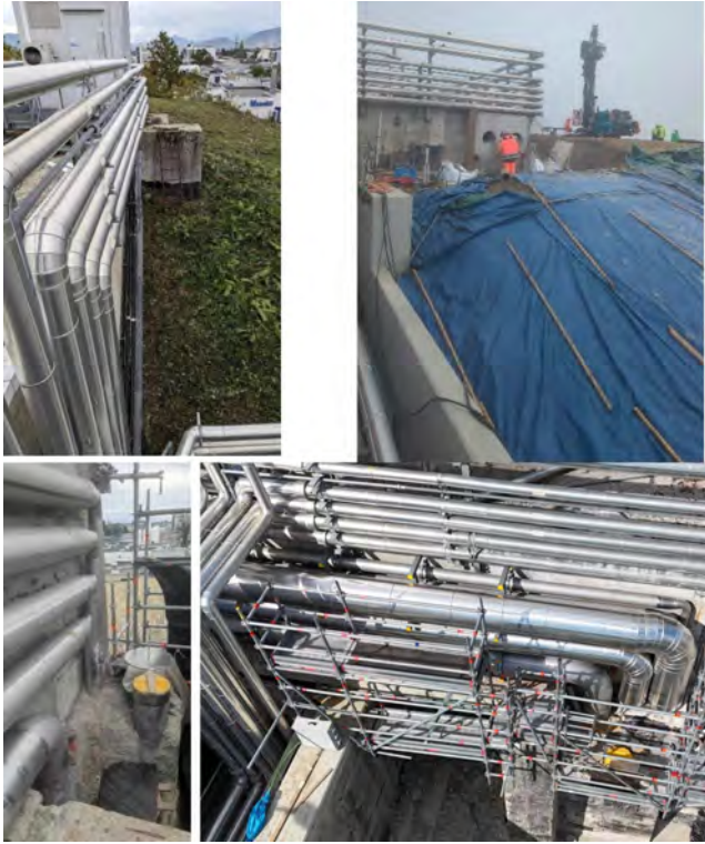
Figure 2: Top left: Concrete shielding structure enclosing the original ventilation ductwork. Top right and bottom left: Demolition of the shielding structure to expose the embedded ducts and pipes. Bottom right: Final configuration after installation and connection of the new steel ducting to the existing infrastructure.
