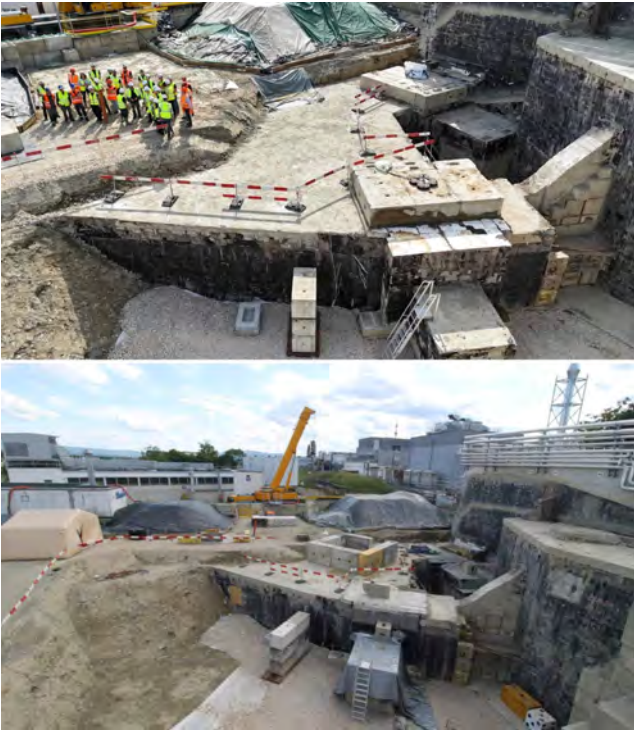
Figure 4: Progress of the IBDRS excavation and dismantling activities. Top: Target area after completion of the soil removal campaign, exposing the civil-engineering infrastructure and surrounding buildings. Bottom: Ongoing dismantling of the beam-dump shielding, showing the infrastructure used for cleaning and handling shielding blocks, together with the crane installed for removal operations.
