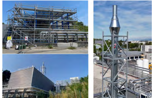
Figure 1: Left: Different phases of the construction of the Building 197 extension, with the top picture showing the internal metallic structure during assembly and the bottom picture the completed building. Right: The 10 m-high ventilation stack installed on top of the new building.
