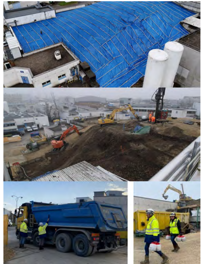
Figure 3: Different phases of the soil removal activities for the IBDRS project. Top: Protective tarpaulin installed over the target area during the final winter months, ahead of excavation work. Middle: IBDRS worksite during the excavation and core-sampling campaign. Bottom left: RP team performing radiological checks on a truck leaving the site. Bottom right: Soil sampling activities for gamma-spectrometry analysis.
