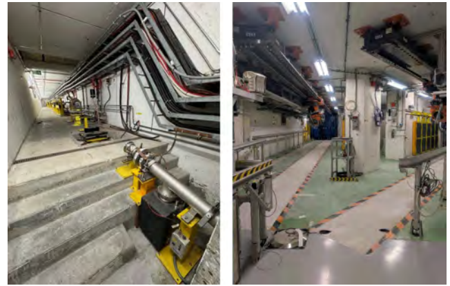
Figure 5: Preparatory activities for the BTY line upgrade during LS3. Left: BTY transfer line on the PS Booster side after the removal of the magnets for refurbishment and consolidation activities. Right: Former ISOLDE robot trenches filled with concrete in preparation for the future installation and handling of the upgraded BTY beamline magnets.
